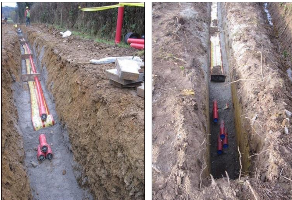
Plate 4-6 Typical Cable Trench View
